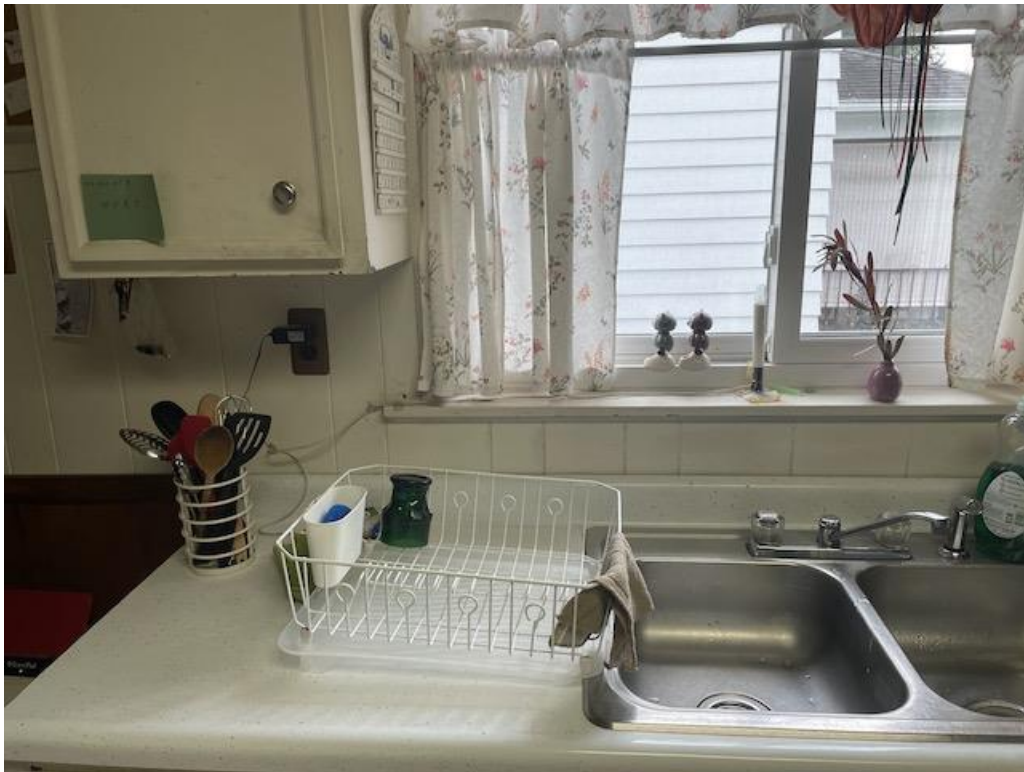
3.2 – No GFCI (Kitchen)
